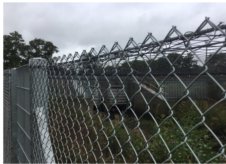
Photo 56: Channel feeds through wastewater treatment plant infrastructure
