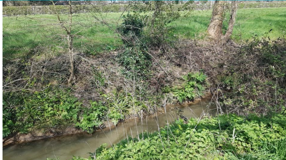
Photo 117: View of left bank at proposed bridge location, low shrubs and saplings on steep banks
