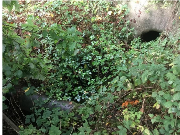
Photo 113: Pipe crossing channel and culvert inlet, heavily shaded and vegetated
