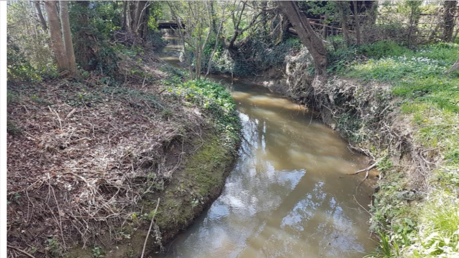
Photo 127: Upstream towards bridge from left bank showing erosion on outer meander bank face and vertical bank profile. Heavily shaded.
