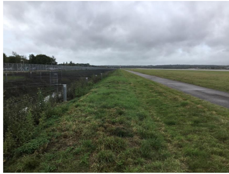
Photo 104: Low embankment on right bank with small breaks
