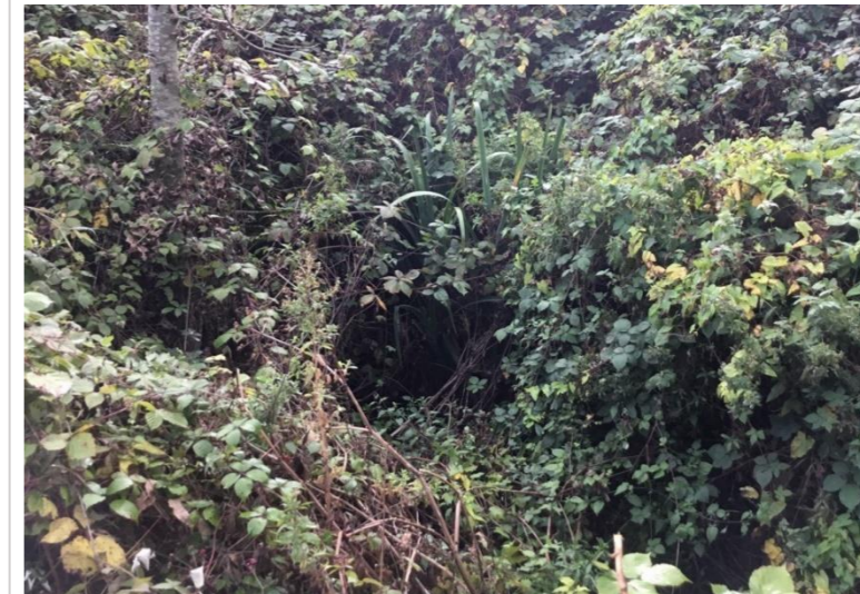
Photo 114: Culvert outlet heavily vegetated
