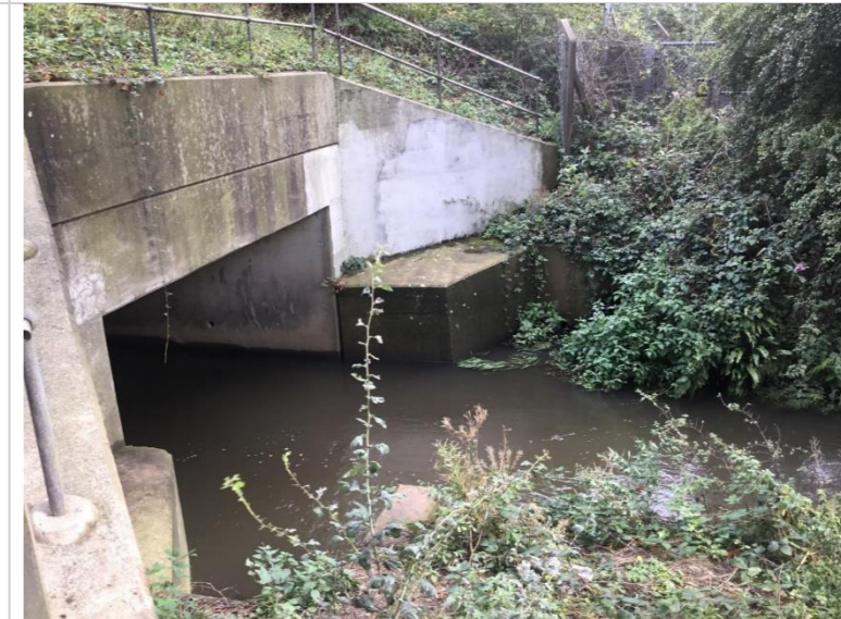
Photo 71: Culvert inlet under Airport Way and London Gatwick Airport shuttle line (outfall on right bank, view obscured by vegetation)
