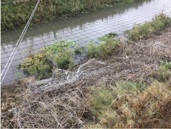
Photo 2: Damaged gabion mattresses
