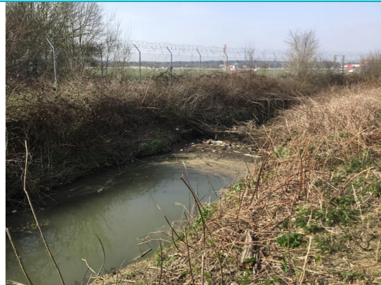
Photo 1: Rubbish caught in old netting at upstream of runway culvert
