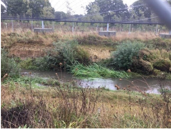
Photo 2: Erosion of vertical right bank and scattered vegetation
