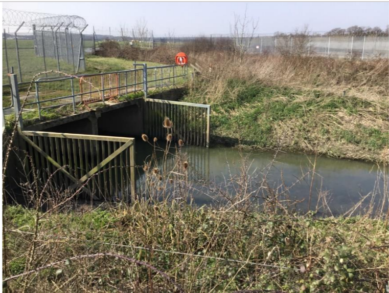
Photo 9: Runway box culvert outlet with security gates open buried in silt
