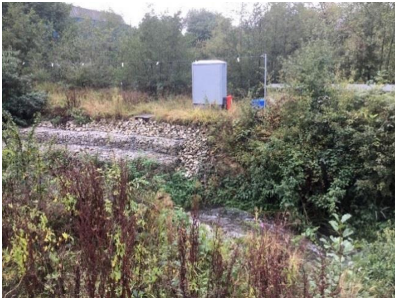
Photo 3: Gabion mattresses and erosion of bank
