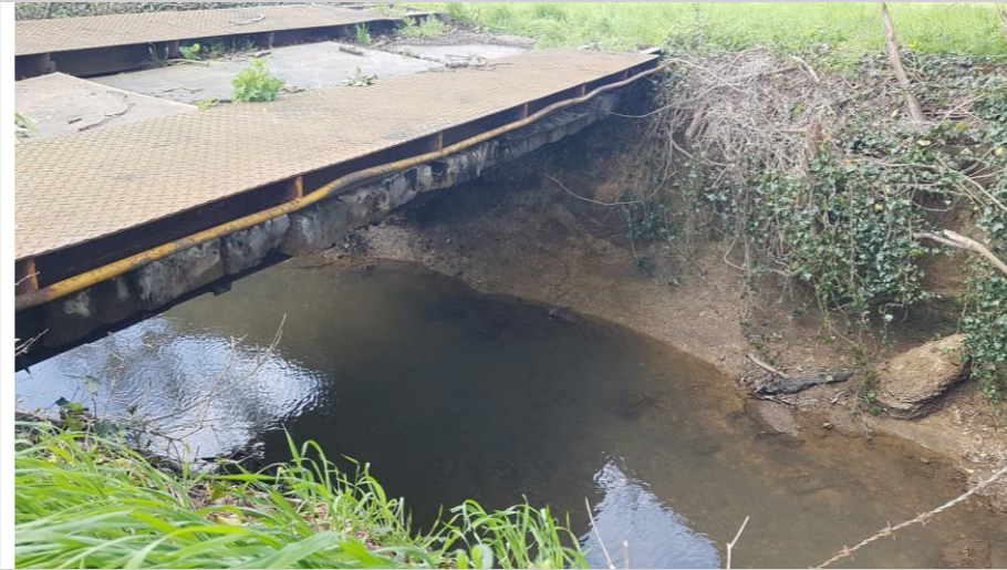
Photo 124: Scour of bed and left bank on outer meander under bridge
